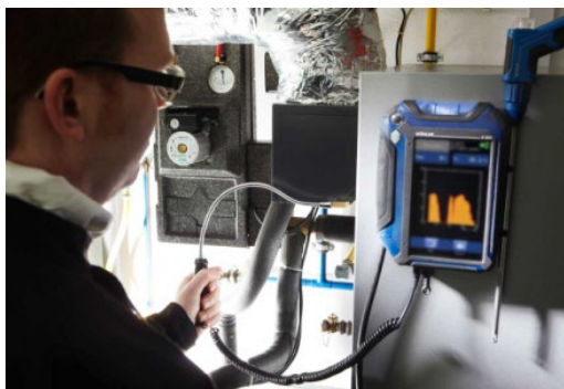
Fig. 45: Spillage test: Searching for condensate
