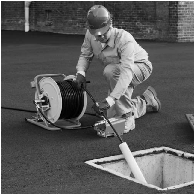
Figure 10 – Extending the Drain Opening to the Operation Point
