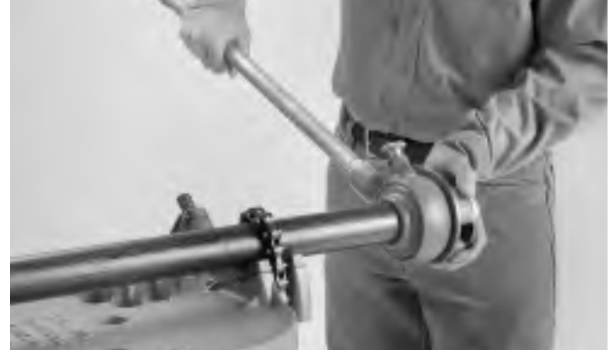
Figure 3 – Sliding Threader On Pipe
